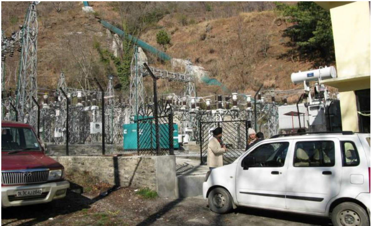
Hydro Power Plant in India.
