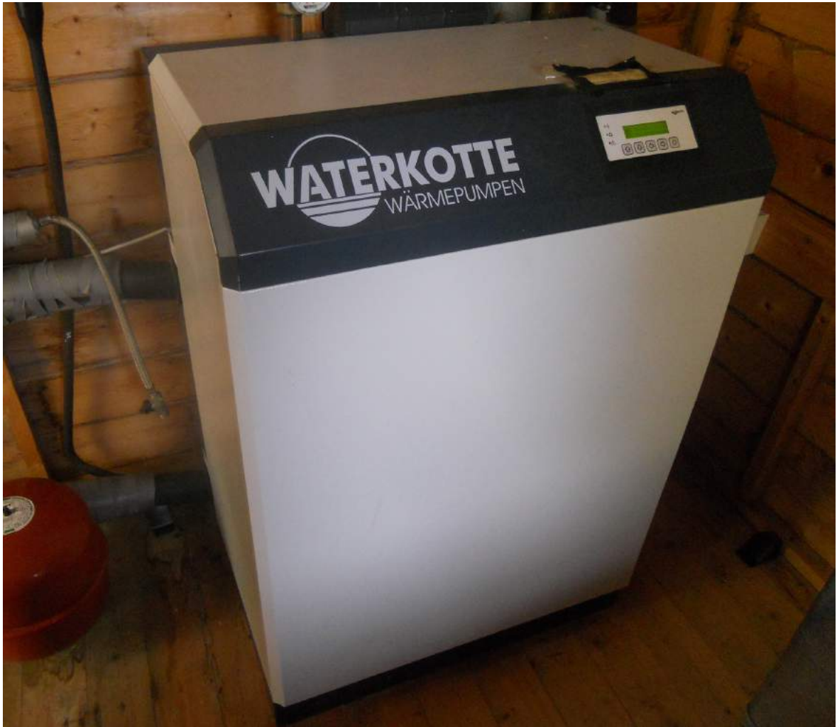
Boiler for Geothermal System of heating the house.
